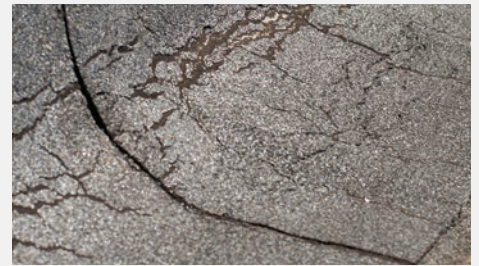
Fix Failing Waterproofing Systems
